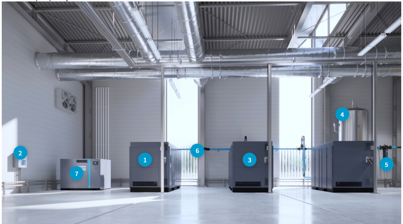
ZR 160-315 (VSD) Compressor Room Installation
