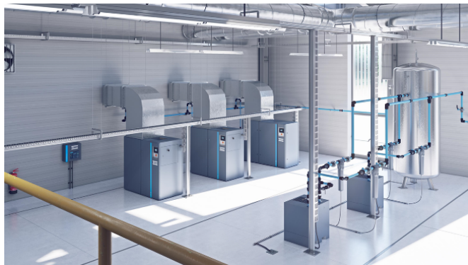
Installation with external dryers
